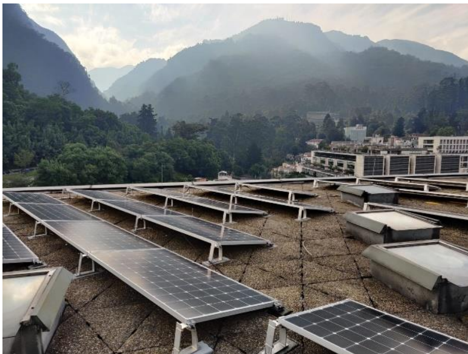
Figure 2. PV installation at SD Building. Bogotá, Colombia
